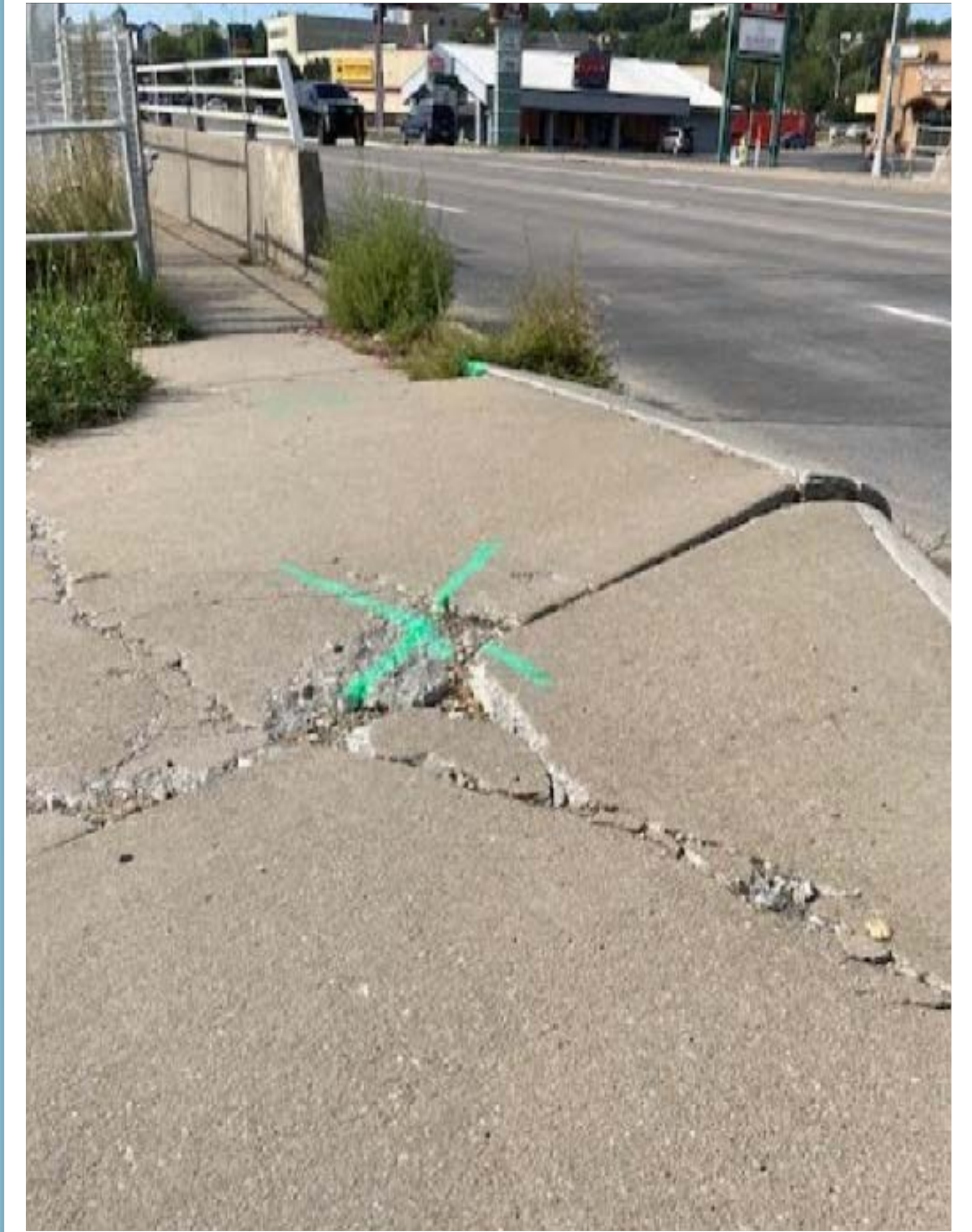
Crumbling concrete on east side of 72nd just north of bridge entrance, facing southwest. Marked with paint by City in July, by September, the property owner had still not been notified.
