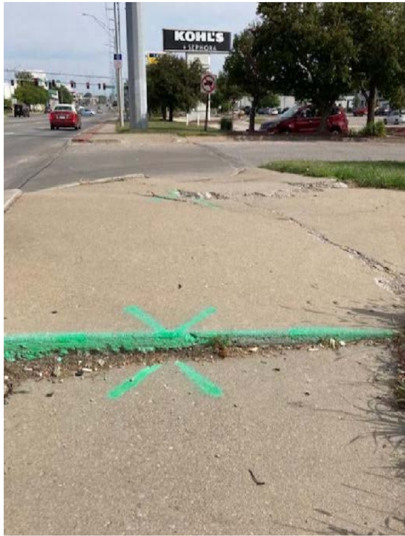
Heaved concrete in the same location as the previous photo, facing north. Marked with paint and barricade by the city in July, by September the property owners were still not notified. The barricade went missing in August and the City was notified.
