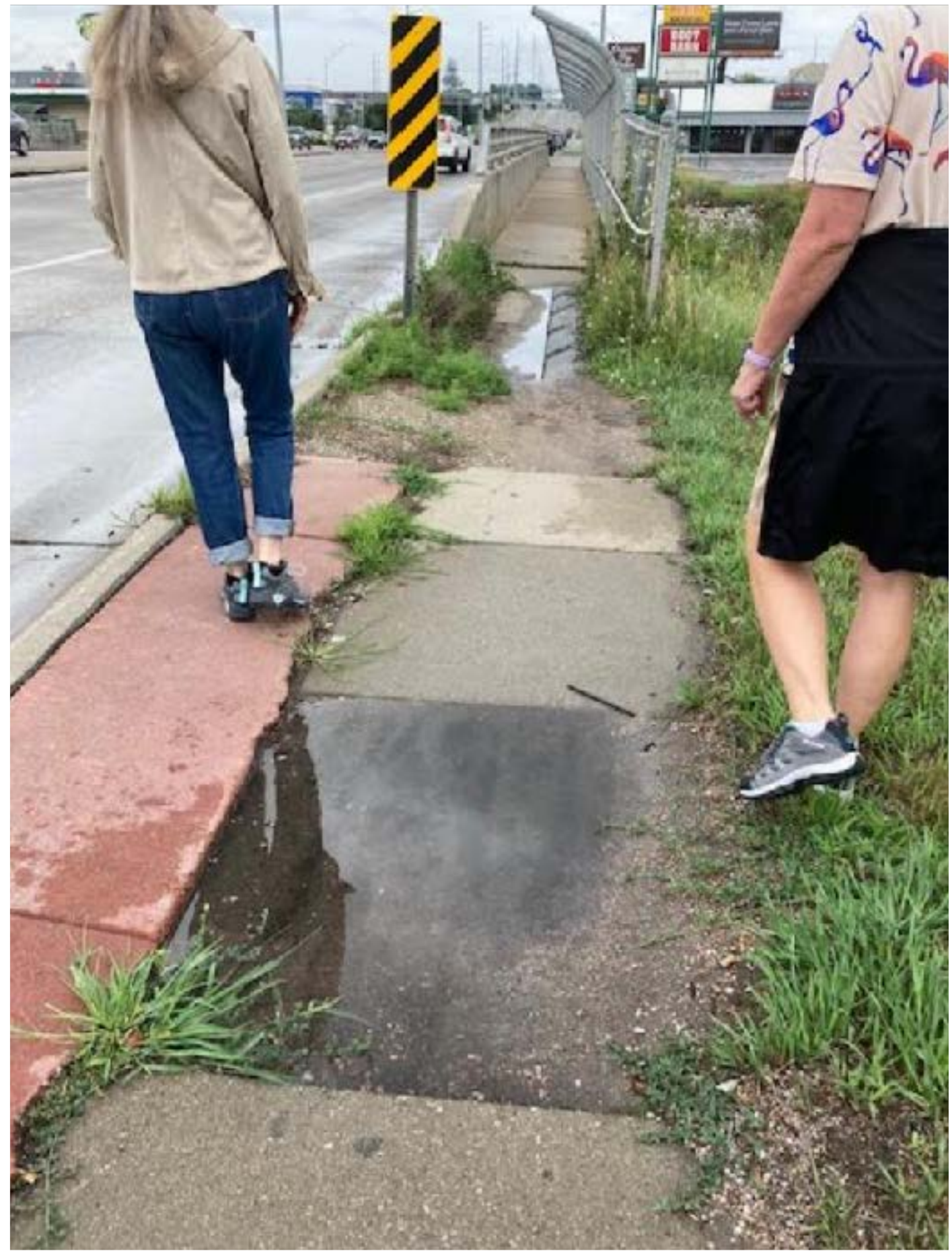
West side of 72nd, south of Rose Blumkin, at the entrance to the bridge - standing water and weeds.
