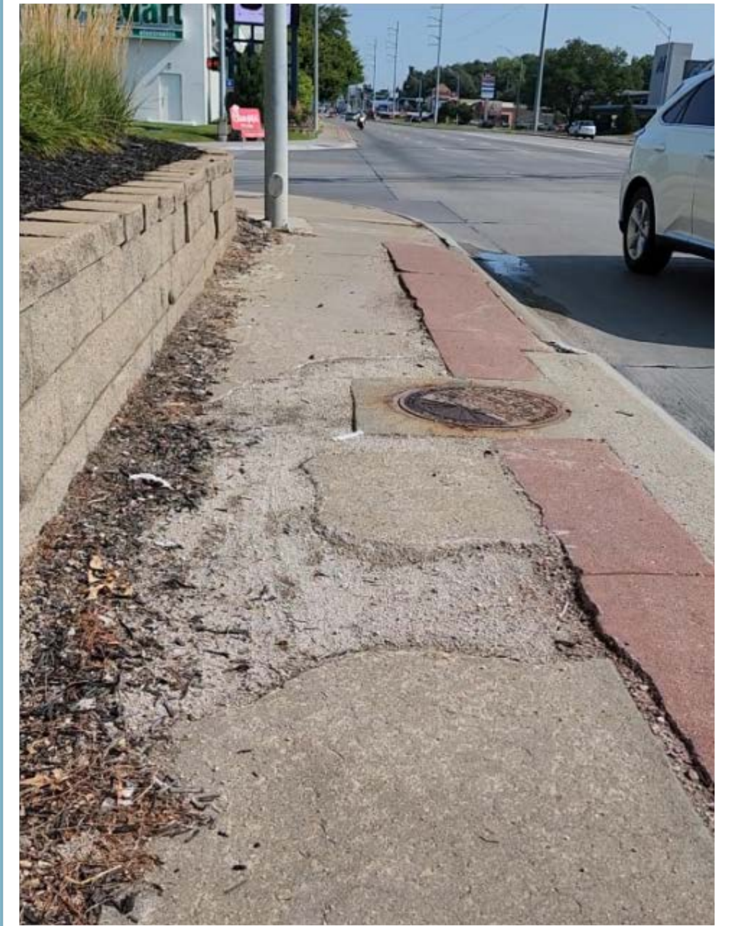
Southwest corner of 72nd & Rose Blumkin - missing/crumbling concrete.
