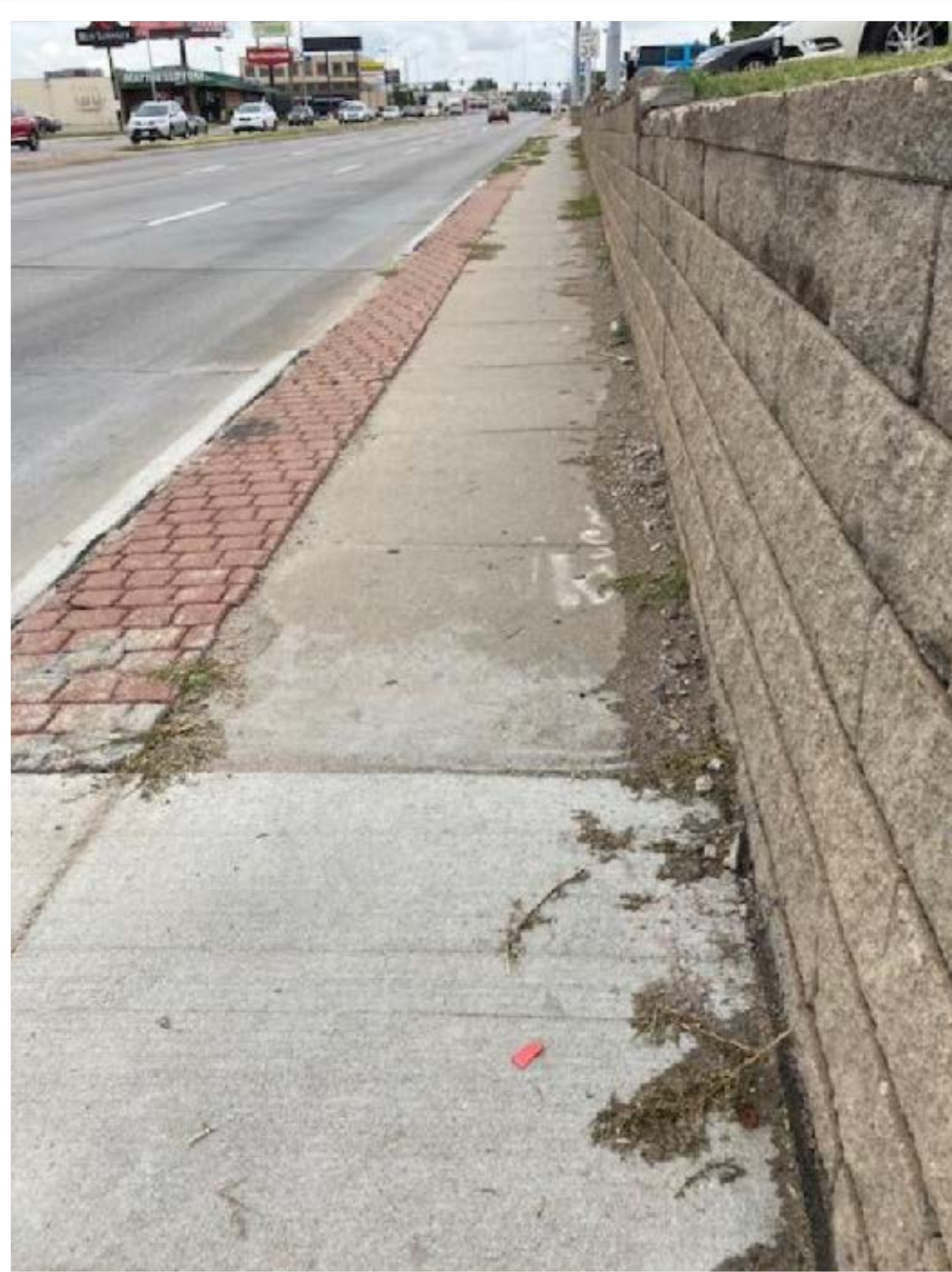
Narrow sidewalk right up against a retaining wall - an area where pedestrians noted not feeling safe (east side of 72nd btwn Jones Circle and Farnam Street)
