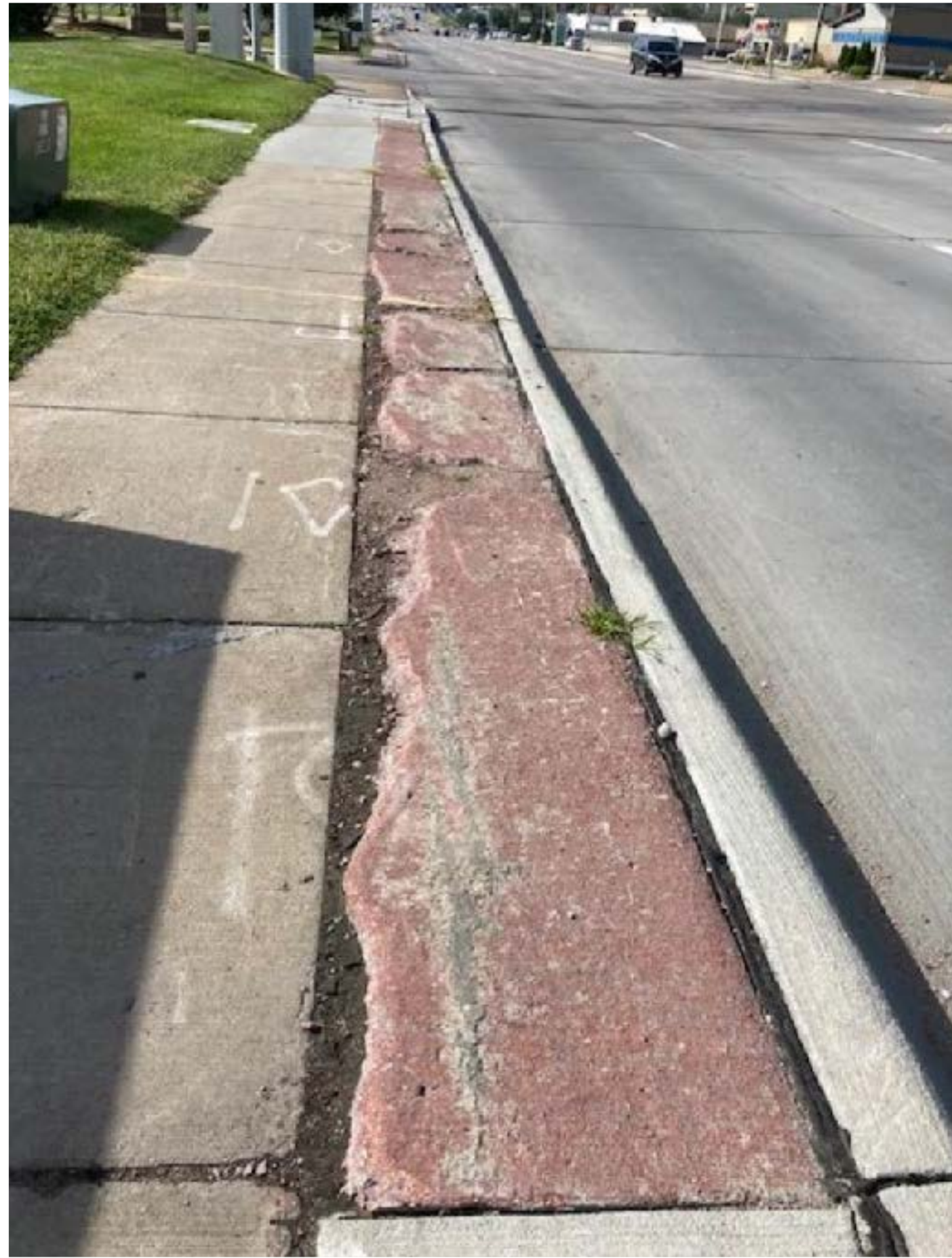
Crumbling concrete on east side of 72nd Street just south of Dodge, looking south.
